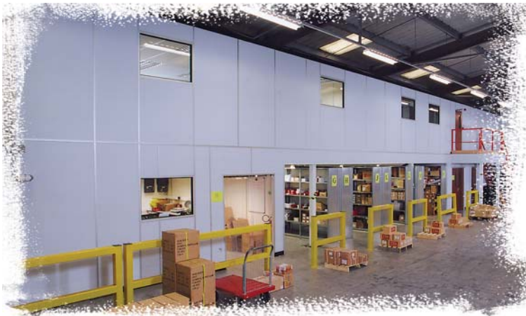
Fire resistant bulkheads integrated with partitioning
